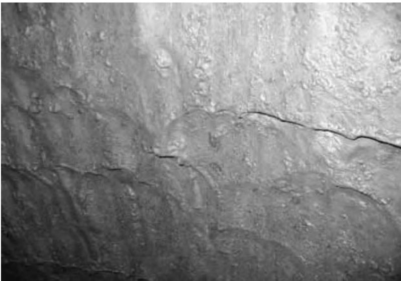
FIGURE 1.5 Refractory surface wear dominated by chemical corrosive (dissolution).
